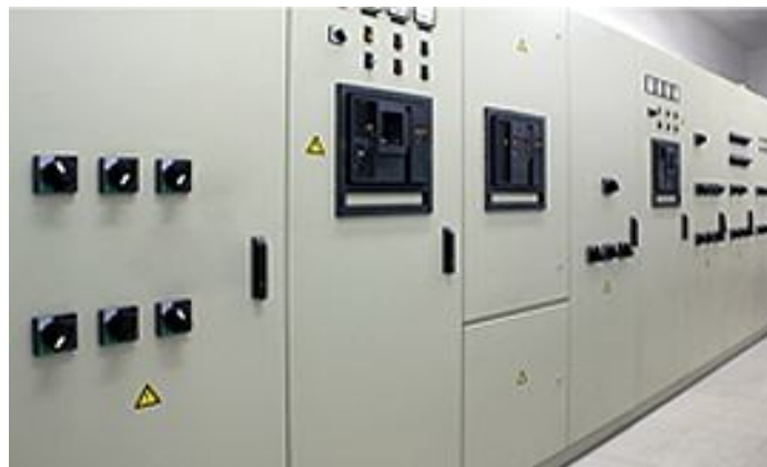
Figure no. 2.4 VFD soft starter panel
